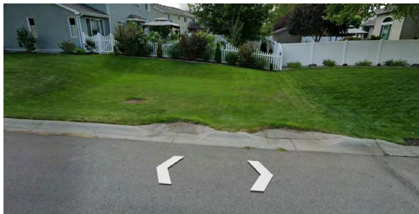
Photo: Example of a Typical Grassy Drainage Swale that has Developed Drainage Issues
